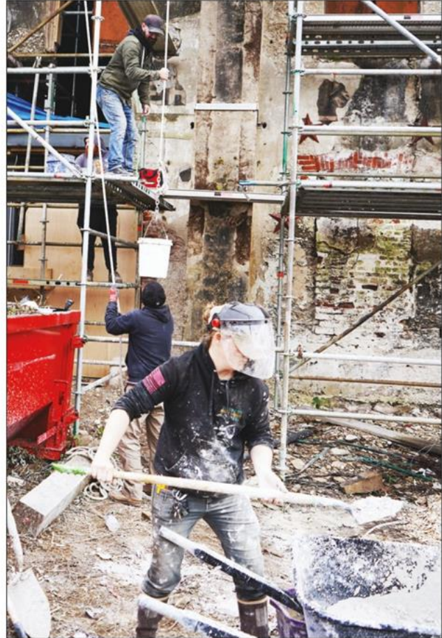
Tabby is shoveled into buckets and hoisted up to the scaffolding, where the tabby is poured into wooden frames. (Photos by Kathleen Russell)
