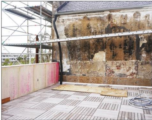
Second floor outdoor seating area will overlook the Darien River. Reproduction slate has replaced the slate roof on the Adam Strain building, which puts less strain on the structure.
