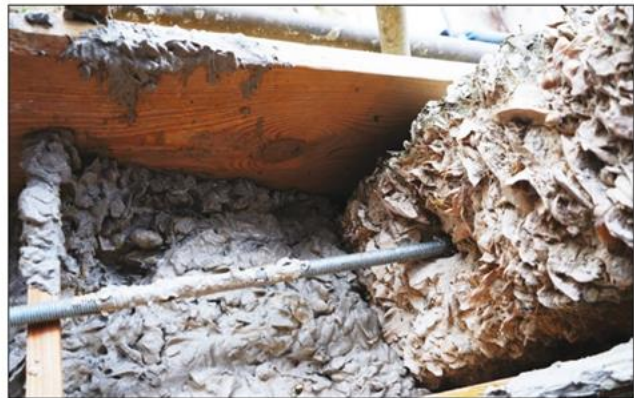
New tabby is shown after it has been poured where it will join with an old section of the original wall.
