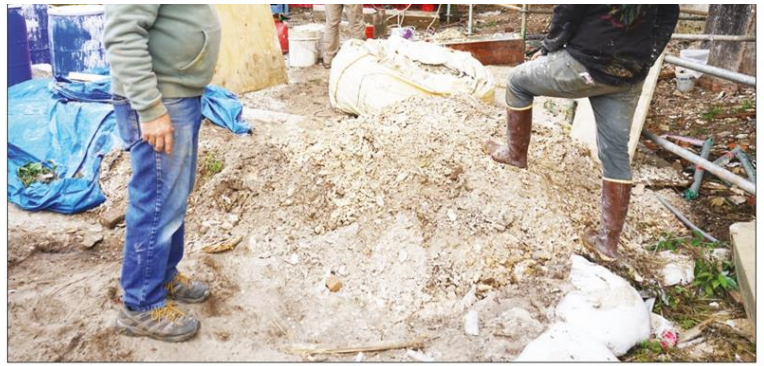
Oyster shells from a crumbling wall of the Adam Strain Building are being reused to rebuild portions of tabby walls of the building. Fred Ecker stands in front of the mound of oyster shells that are to be washed before being used to create the tabby.
