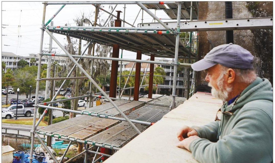
Fred Ecker, project manager for Landmark Preservation, overlooks the restoration of the 209-year-old historic Adam Strain building on Broad Street in Darien. (Photos Kathleen Russell)
