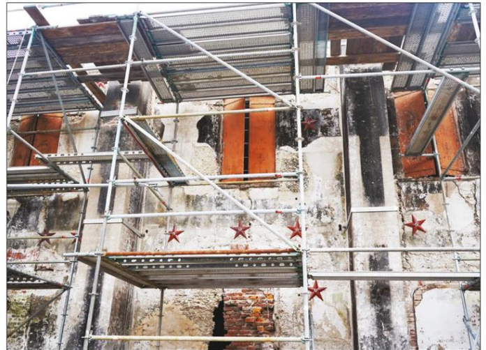
Exterior Patress plates (stars) with rods attached to interior steel beams provide a support system for the exterior walls of the Adam Strain Building. (Photos by Kathleen Russell)
