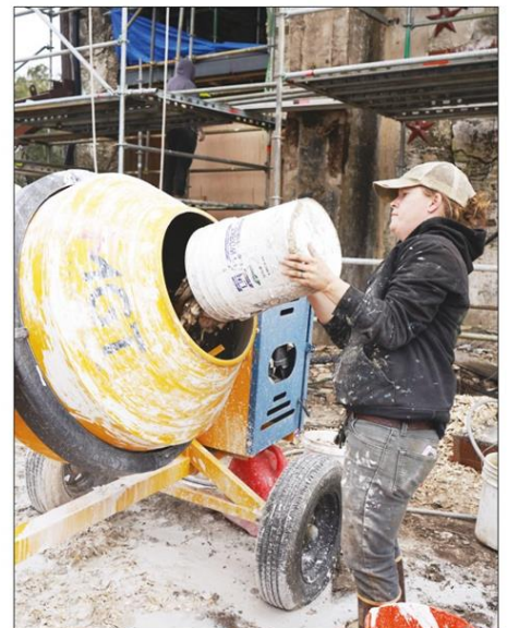
Left photo: oyster shells for a crumbling tabby wall are being washed before recycled to create more tabby. Above photo: the recycle oyster shells are
